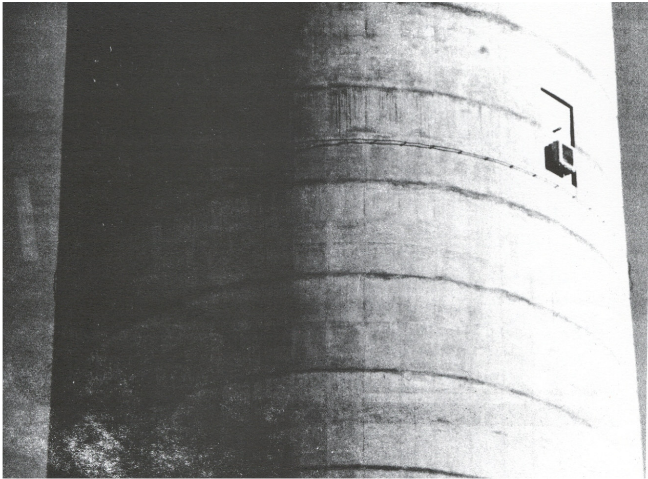
Figure 14-2. High-intensity obstacle lights installed on a chimney
